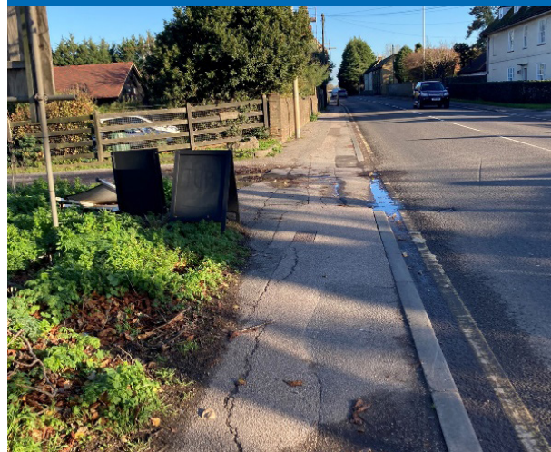
Narrow and uneven footway
