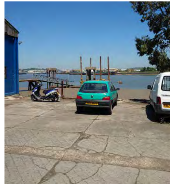
The hard concrete edge where the lanes meet the river.
