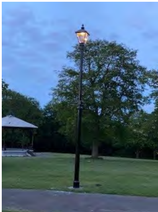
Heritage solar lamp column at Victoria Gardens
