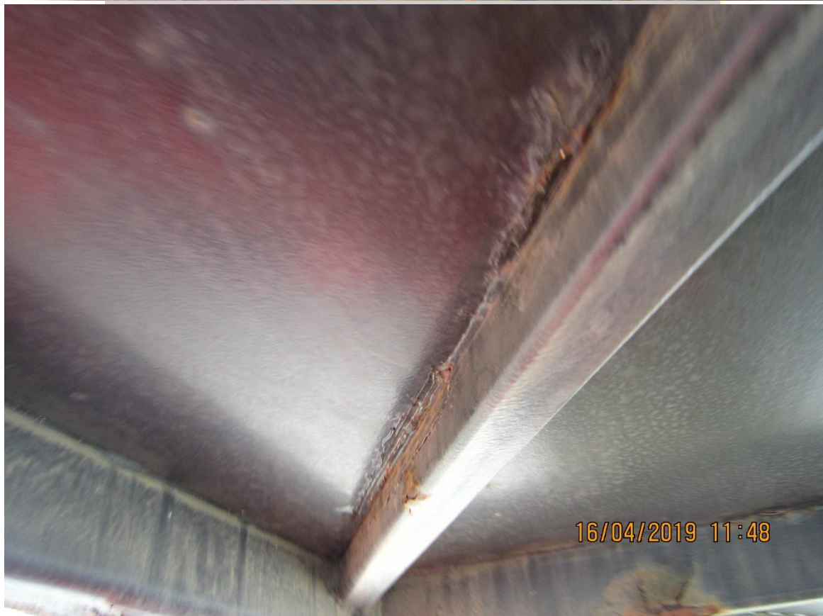
These are all water traps between deck and bottom stringer, where deck is stitch welded.
