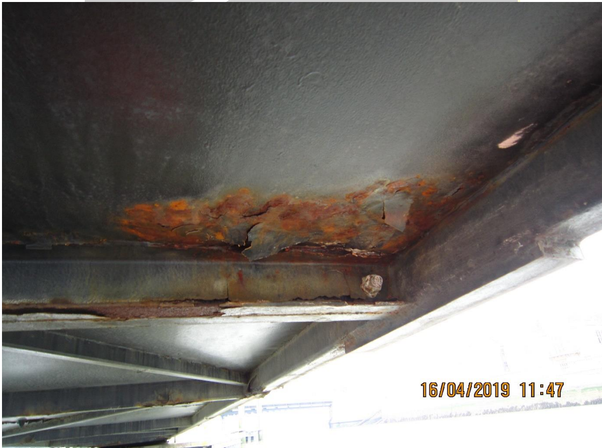
Channel joint, in middle of brow where brow was joined after fabrication and road haulage.
