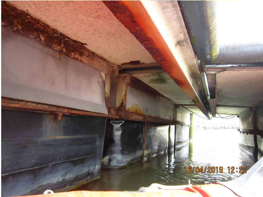
View through front to back. Note corrosion heaviest at front and non-existent at rear.
