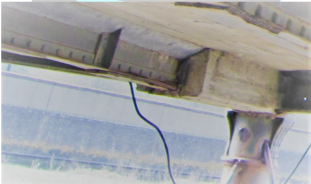
2019 photo blown concrete patch crack has expanded and will eventually fall away.
