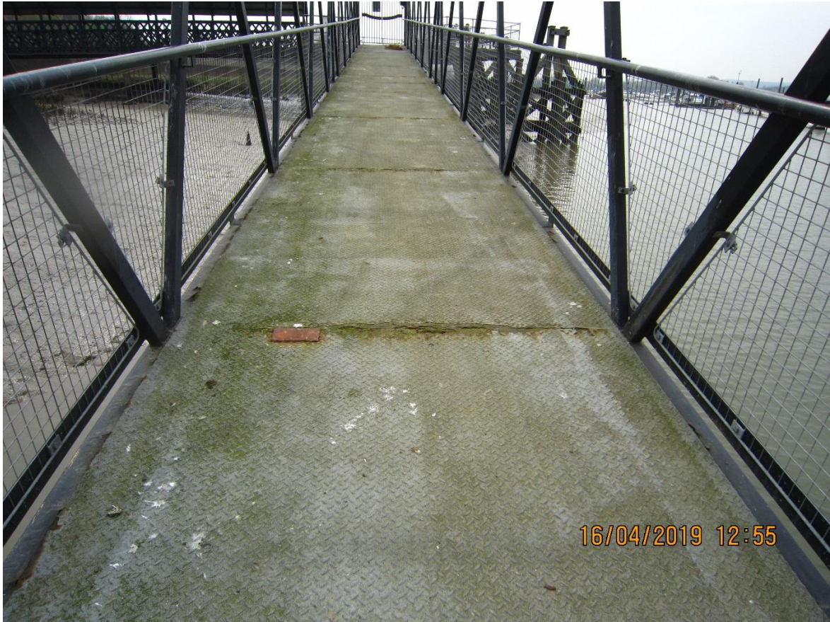
There are repairs of areas, areas with deck cut out and plate welded over cut out and patches welded over holes and holes. 2No. visible holes as of survey.
