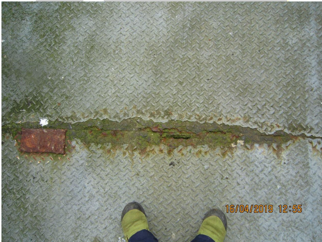
view of patch and hole.
