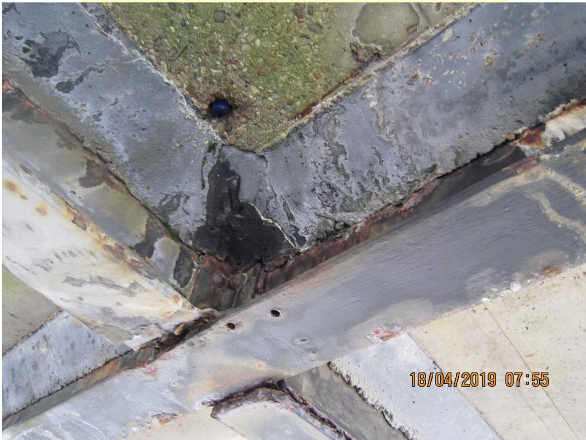
Photo from 2019 of same area. Corrosion continuing and repairs are becoming redundant.
