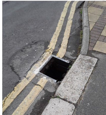
Missing Gully Cover reported as emergency
