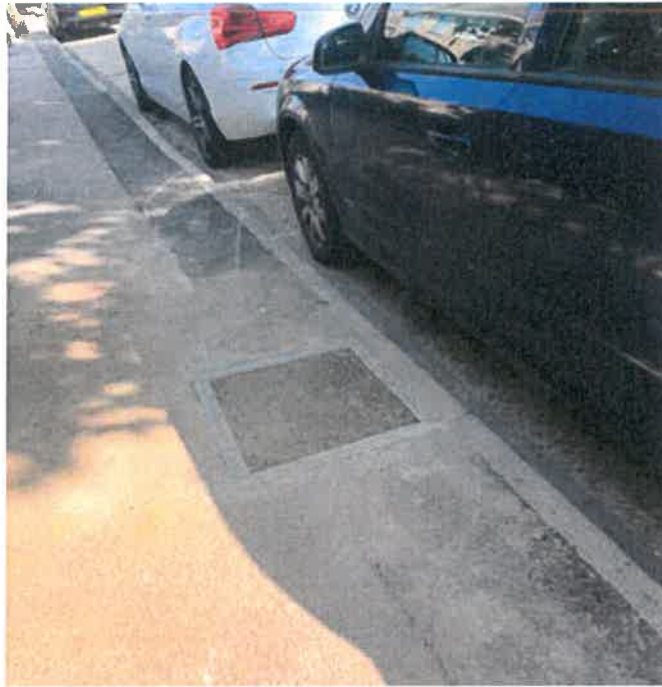
A tree pit created at no cost during collaborative working with cable laying Lanes-i
