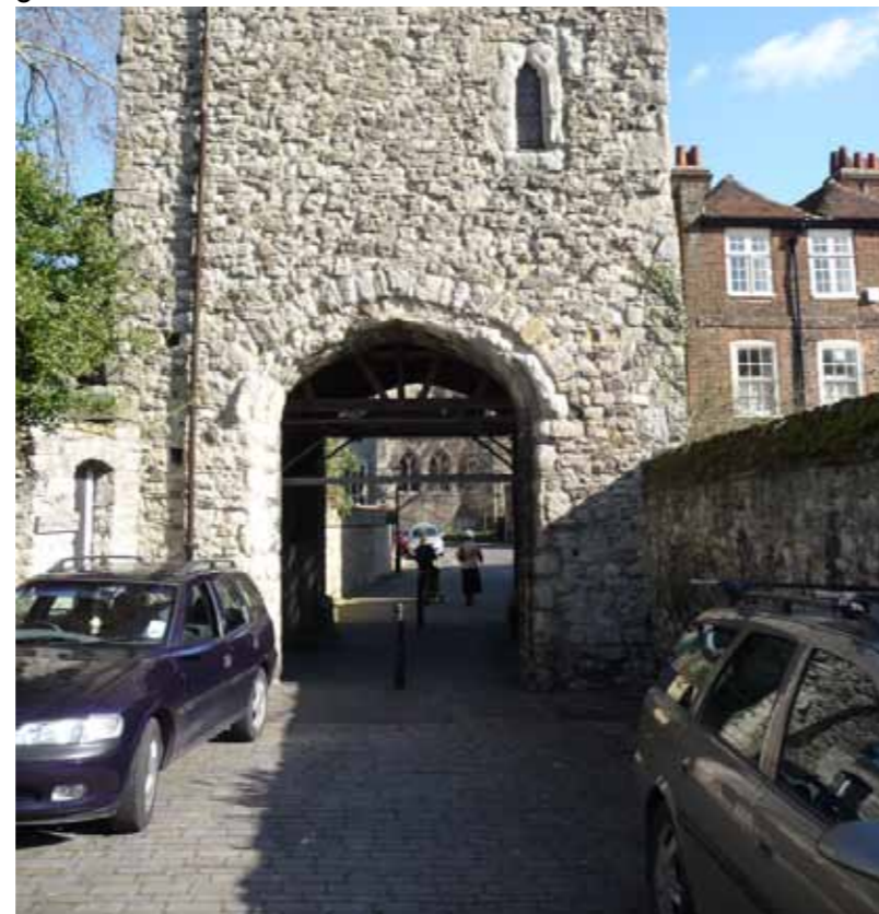
Fragments of rag-stone pitching to the front of Priors Gate
