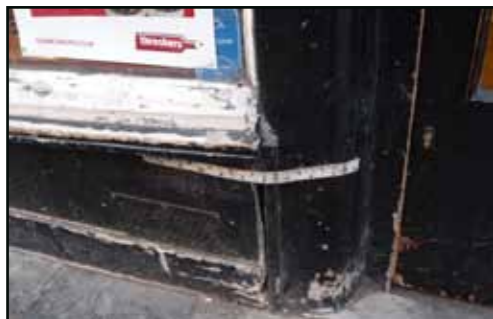
Examples of deterioration
