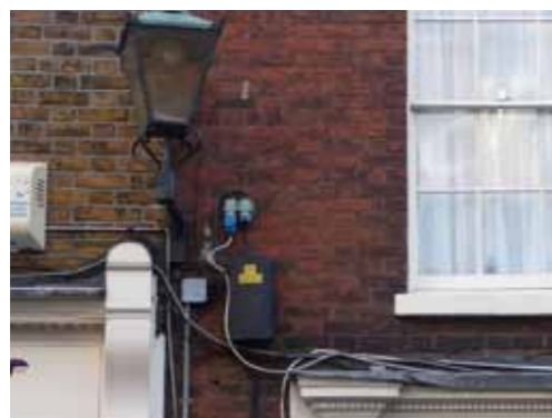
Ad-hoc accumulation of wires
