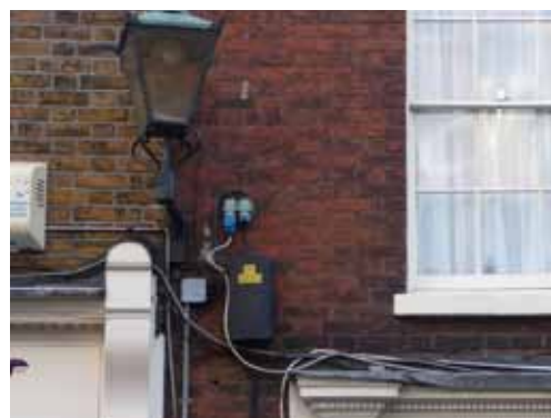
Ad-hoc accumulation of wires
