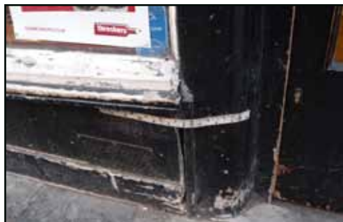
Examples of deterioration
