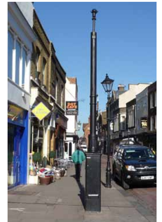
CCTV post-top camera
