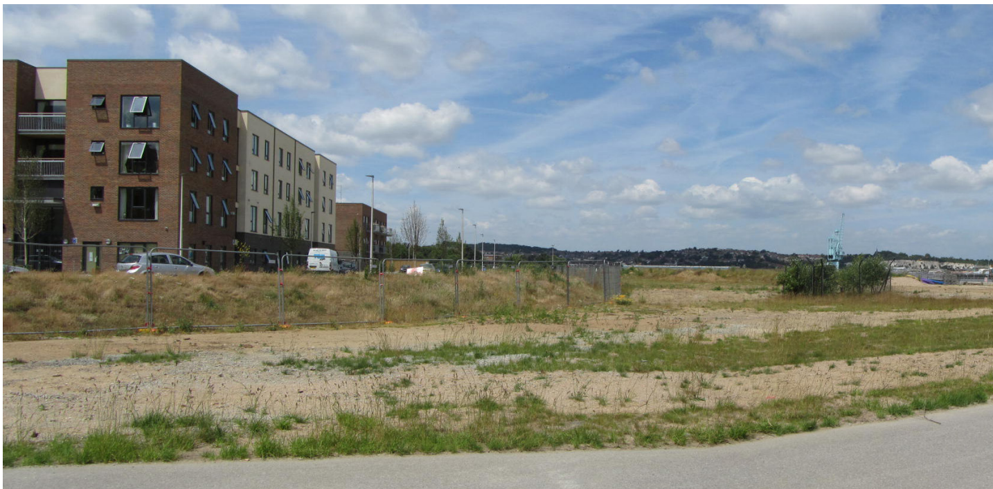
View towards Stanley Wharf which will be the second phase of development
