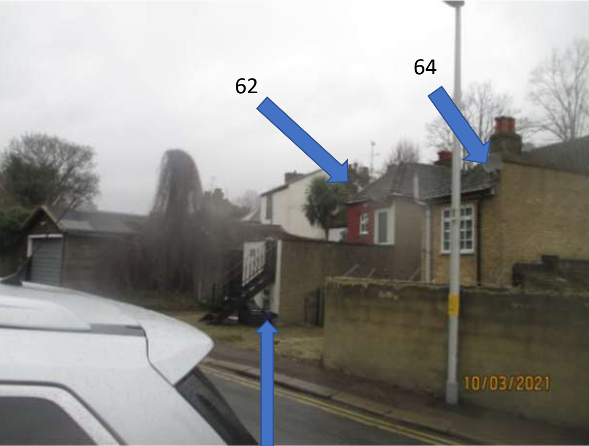
Close ground floor window obstructed by stairs
