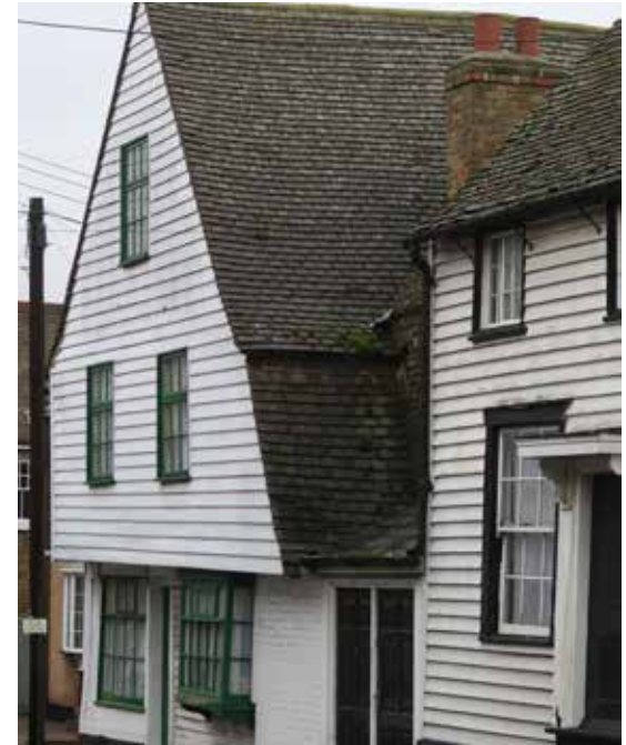
Figure 56: Longford House, a Grade II listed building with jettied upper storeys and painted window frames.
