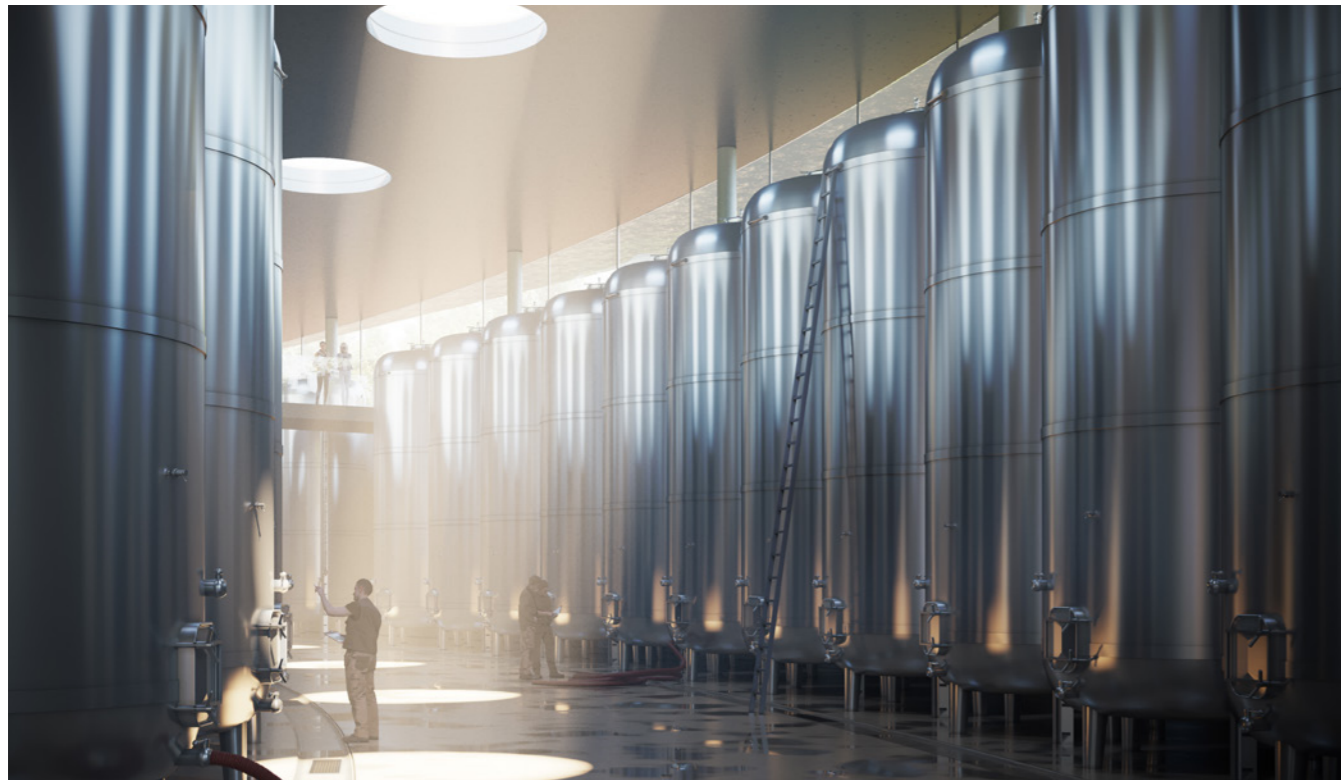
Over 70% of the building is dedicated to wine making, including the processing facility on the lower ground floor
