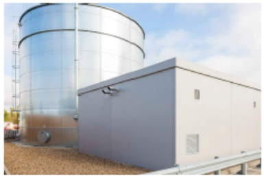
Typical Sprinkler Tank & Pump House Image
