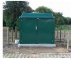
Typical Sub-Station Image
