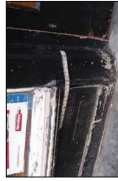
Examples of deterioration
